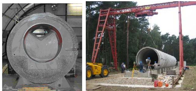
Figures 2: Mock-ups for backfill tests with grout. LEFT: small-scale mock-up after slicing. RIGHT: construction of 30 m long large-scale mock-up
