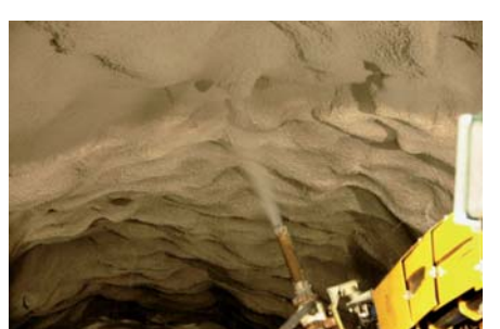
Large scale field test using low pH shotcrete for rock support at the Hagerbach underground facilities
