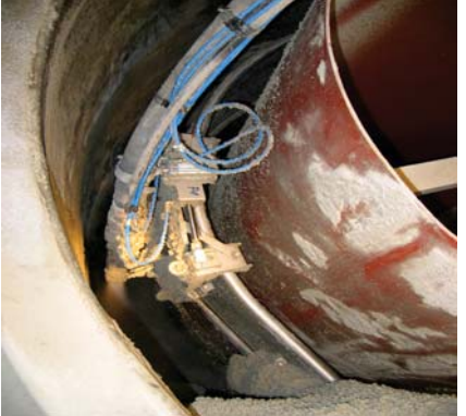
Granular materials backfill placement machine and spray nozzle during test with MX-80 Bentonite at Mol
