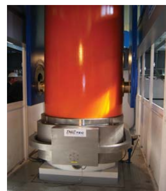
Transfer cask docked onto the borehole lock ready for emplacing BSK-3 canister into the borehole
