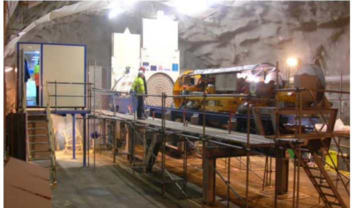
Figure 9: Water Cushion Emplacement Machine with 45 Ton Super Container in Background (SKB / Posiva)
