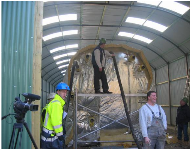
Figure 2: End of the grout injection test (picture taken April 8 th 2008 at 18:20 pm)
